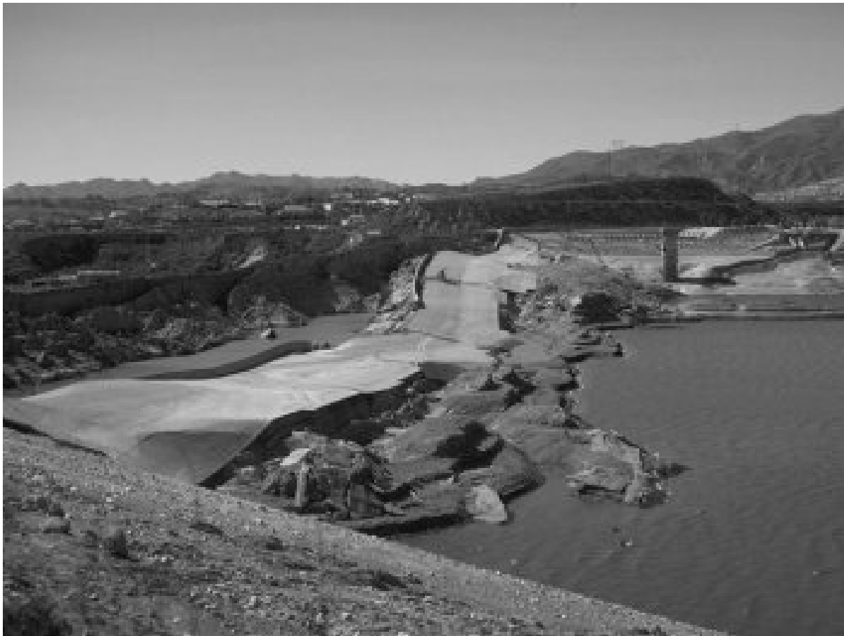
Figure 2-16: Portion of Lower San Fernando Dam That Experienced Flow Liquefaction Following 1971 San Fernando Earthquake (Courtesy of EERC, Univ. of Calif.)
