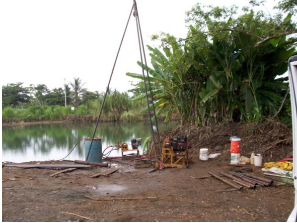
Photo 3: View of the site of borehole P-1 at the Rio Bananito Highway Bridge. The borehole is on the right margin of the river.
