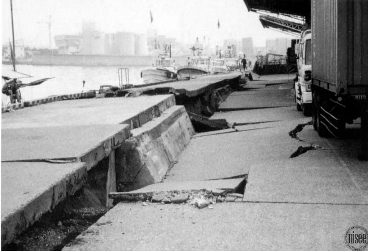
Figure 2-15: Graben Formed Behind a Displaced Quay Wall in Kobe, Japan Following 1995 Hyogoken-Nanbu Earthquake (Courtesy of NISEE, Univ. of Calif.)
