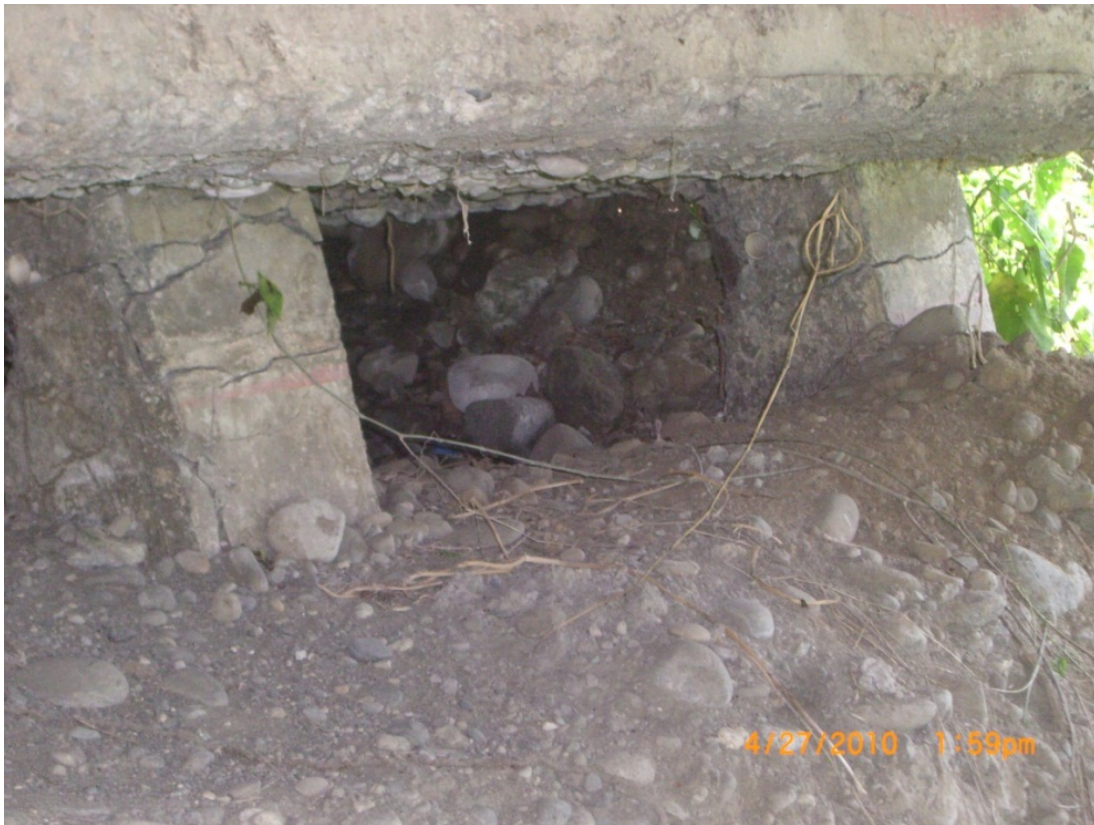
Figure 8-5: Pile Cracking Observed at the East Abutment of the Rio Cuba Bridge
