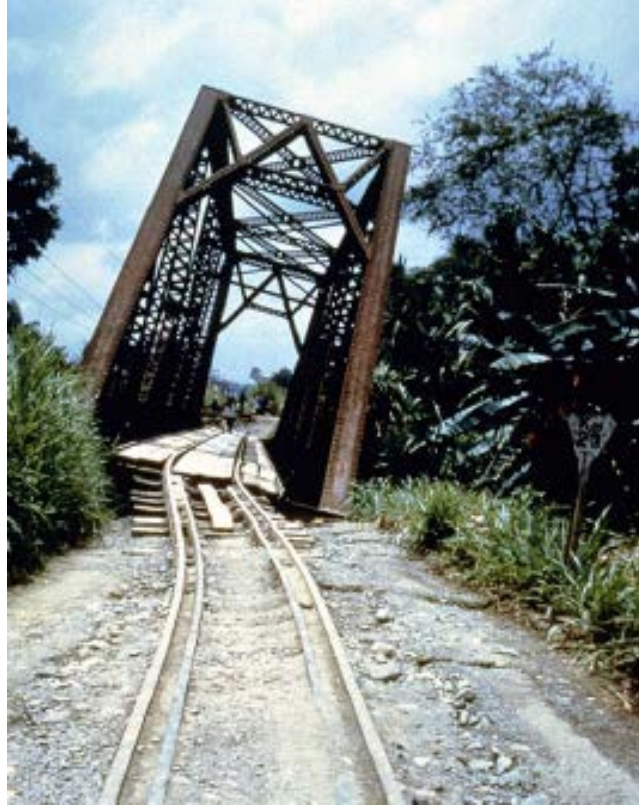
Figure 11-5: Damaged Rio Bananito Railway Bridge Following the 1991 Limon Earthquake (After Youd, 1993)
