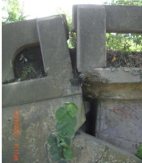
Figure 9-2: Rotation of the Pile Cap at the East Abutment of the Rio Blanco Bridge
