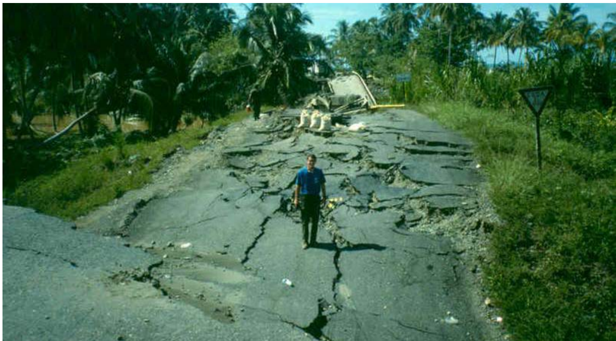
Figure 10-3: Liquefaction Deformations at the South Approach Embankment for the Rio Bananito Highway Bridge
