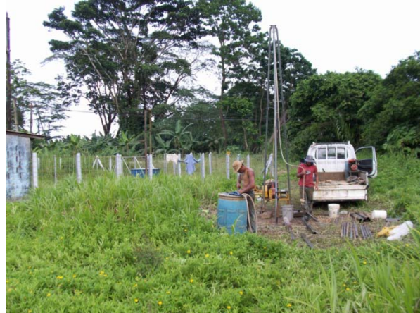
Photo 6: View of the site of borehole P-2 at the Rio Bananito Railroad Bridge. The borehole is about 15 – 20 m apart from P-1.
