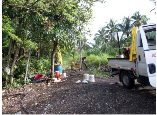
Photo 4: View of the site of borehole P-2 at the Rio Bananito Highway Bridge.
